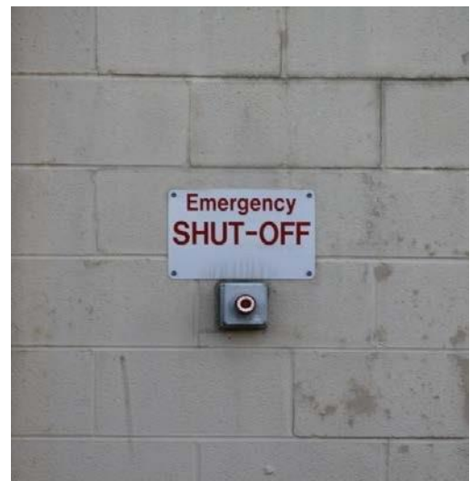
Emergency Shut Off for Maryville Fueling Station
