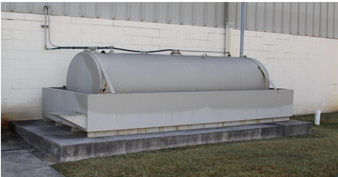
Storage with Secondary Containment
