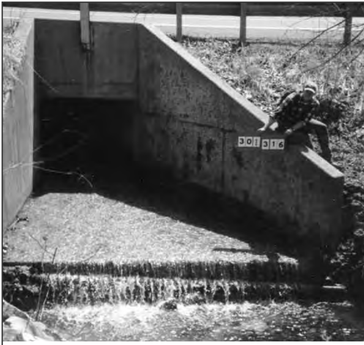
Figure 4.6.5-1. Perched culvert causing fish migration blockage.
