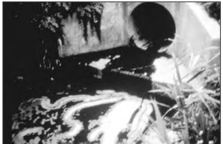
Figure 4.6.4-2. Example of a severe pipe outfall.
