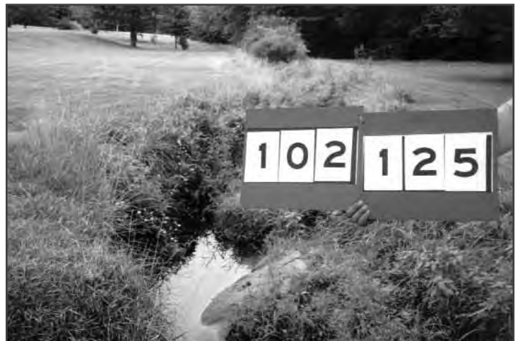
Figure 4.2-1. Photograph showing site number board at a site with an inadequate stream buffer.
