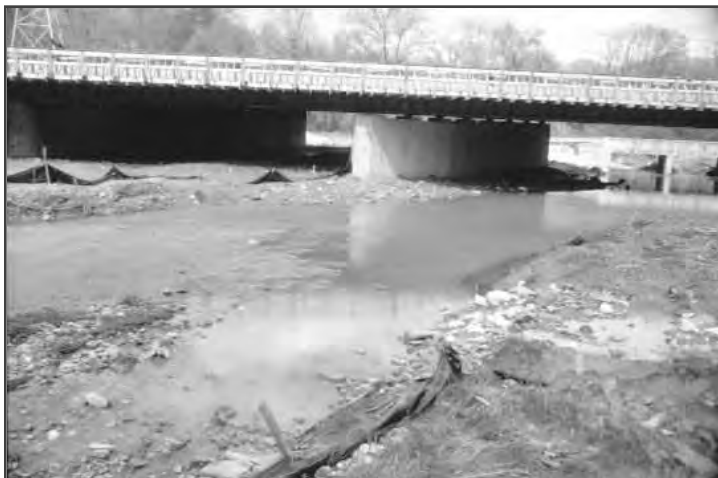
Figure 4.6.7-2. Example of severe construction site where sediment control fencing has failed
