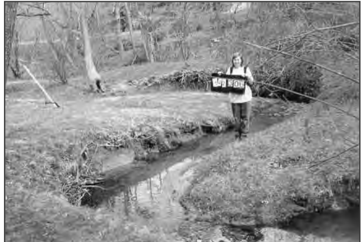
Figure 4.6.2-3. Example of a minor eroding stream bank problem.
