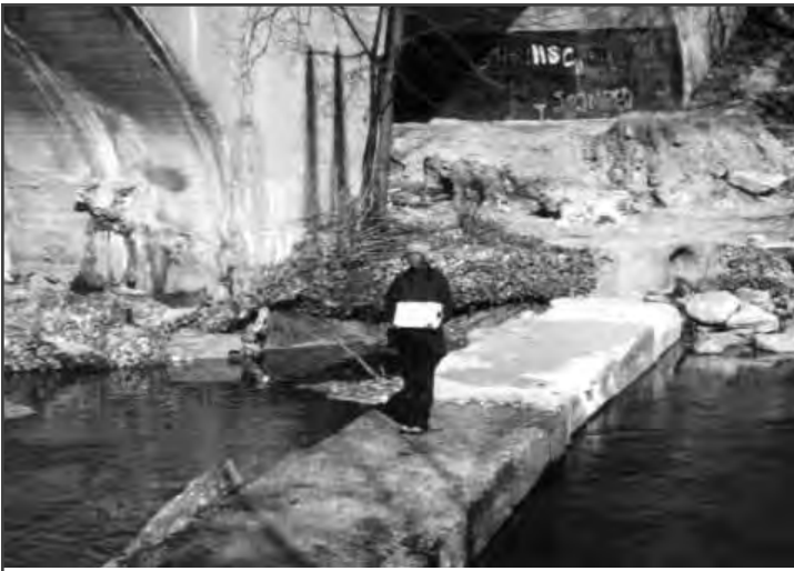
Figure 4.6.3-2. Example of a sever exposed pipe problem.
